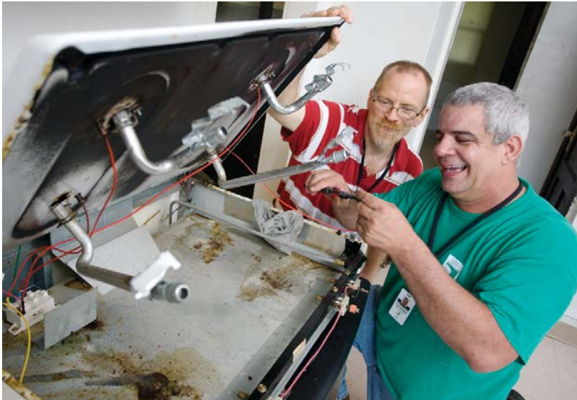
Randy Good (left) and maintenance technician Carlos Berdellans work on a stove top range in one of the Anawim Housing units.
